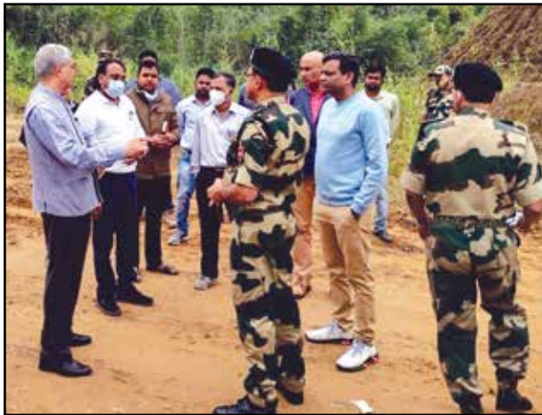
Review of Eastern Border Fencing site by Secretary, Border Management & Joint Secretary, Inspector General, Border Security Force along with officers of NPCC
